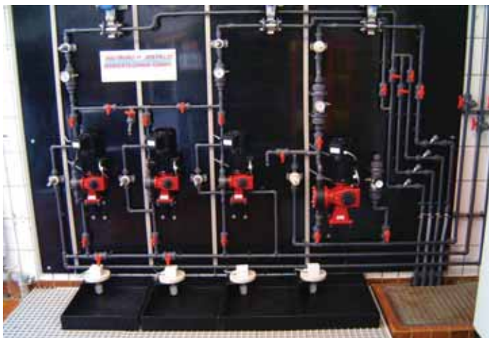
The dosing station (with MEMDOS E) at Fürstenfeldbruck WWTP began operation at the beginning of 2005.
