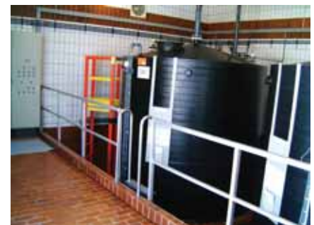
Tank 1 of wastewater treatment plant Fürstenfeldbruck.
