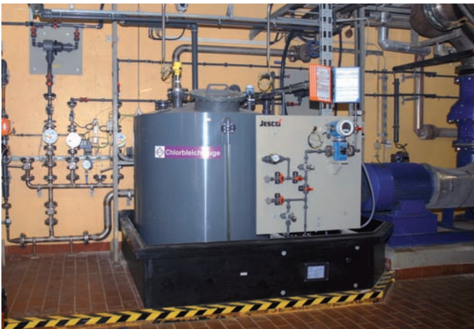
Customer-specific dosing systems in industrial waste water treatment
