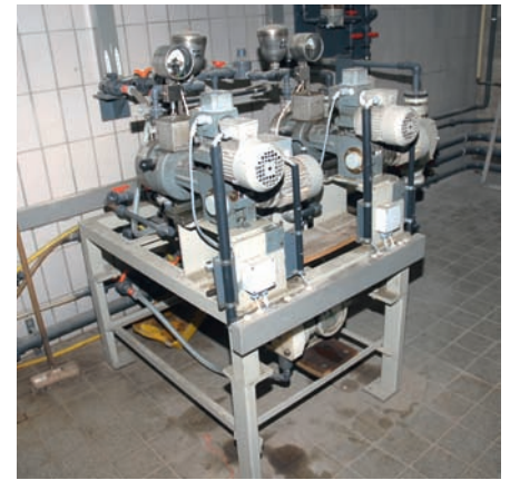
Old treatment plant with JESCO dosing pumps
