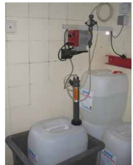
A solenoid driven dosing pump MAGDOS LT is applied in conjunction with the multi-function valve PENTABLOC for the adjustment of pH value.
